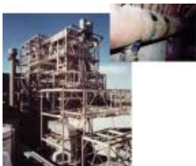
図1 適用対象例(発電ボイラ) Fig. 1 An application example of fatigue sensing technology (Boiler)
